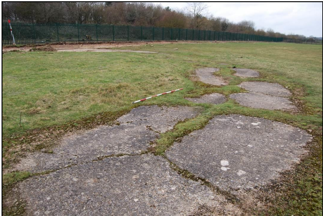
Plate 5: Cracked Concrete Disposal Loop Looking West
