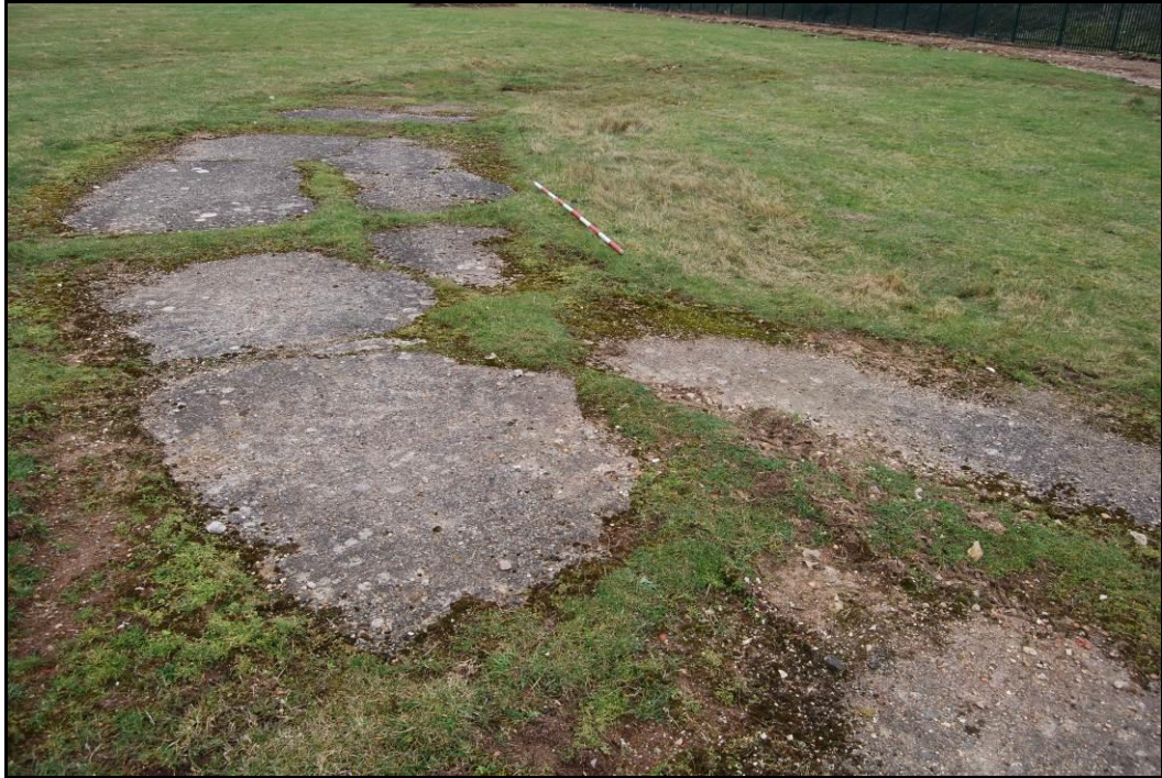
Plate 6: Cracked Concrete Dispersal Loop Looking Southeast
