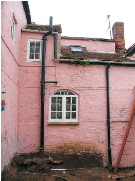
SOUTH WEST FACING SHOT OF THE AREA OF PROPOSED DEVELOPMENT. SOME REDUCTION OF THE GROUND LEVEL ALREADY UNDERTAKEN.
