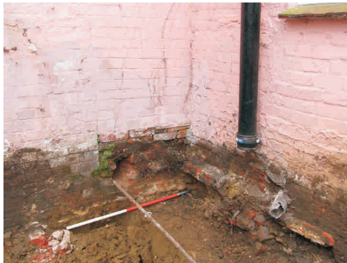
SOUTH FACING SHOT SHOWING INITIAL REDUCTION OF GROUND LEVEL IN THE AREA OF PROPOSED DEVELOPMENT
