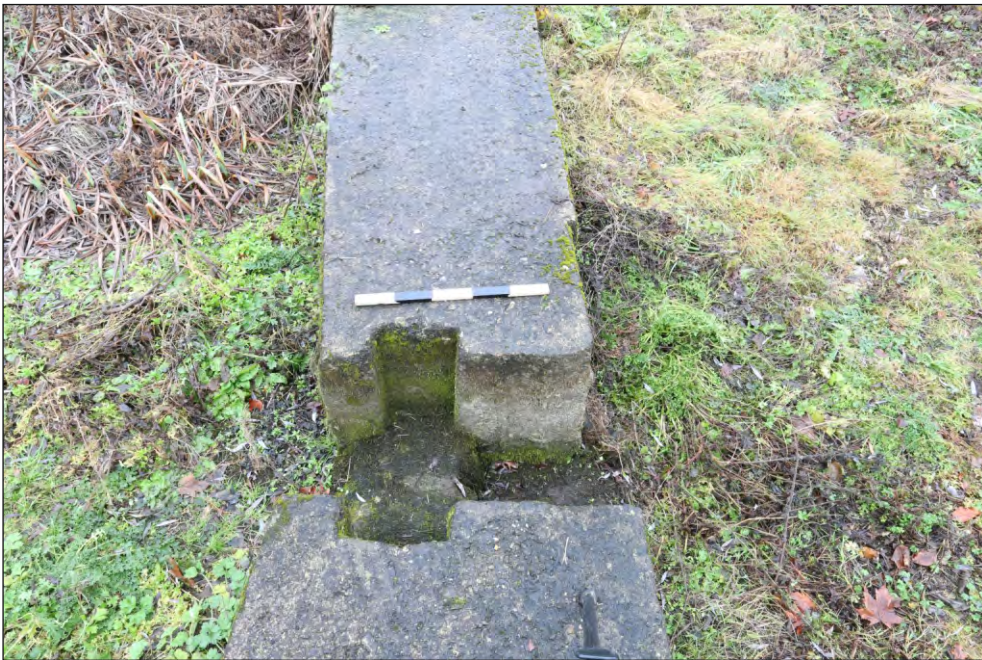
Plate 10: The central gap in Weir 2 viewed from above. The wider slot and vertical grooves to the right of it likely indicate the position of sluice gates to control the flow of water.
