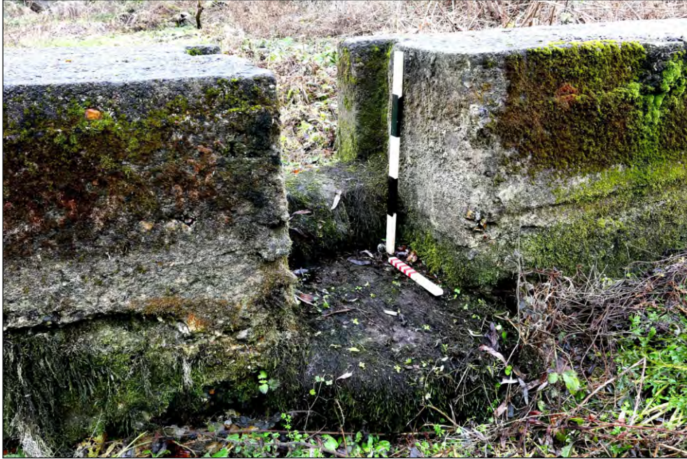
Plate 11: The central gap in Weir 2 viewed from the south-east, showing the change in level and vertical grooves inside it.
