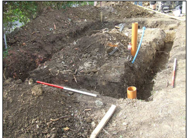
Plate 2: Excavation area of new build and footing trench, looking NW ( scale 2x1m )
