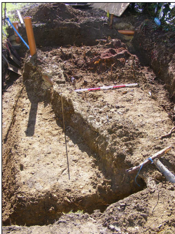
Plate 3: New toilet area excavated a further 300mm exposing limestone surface towards the east, looking S ( scale 1m )
