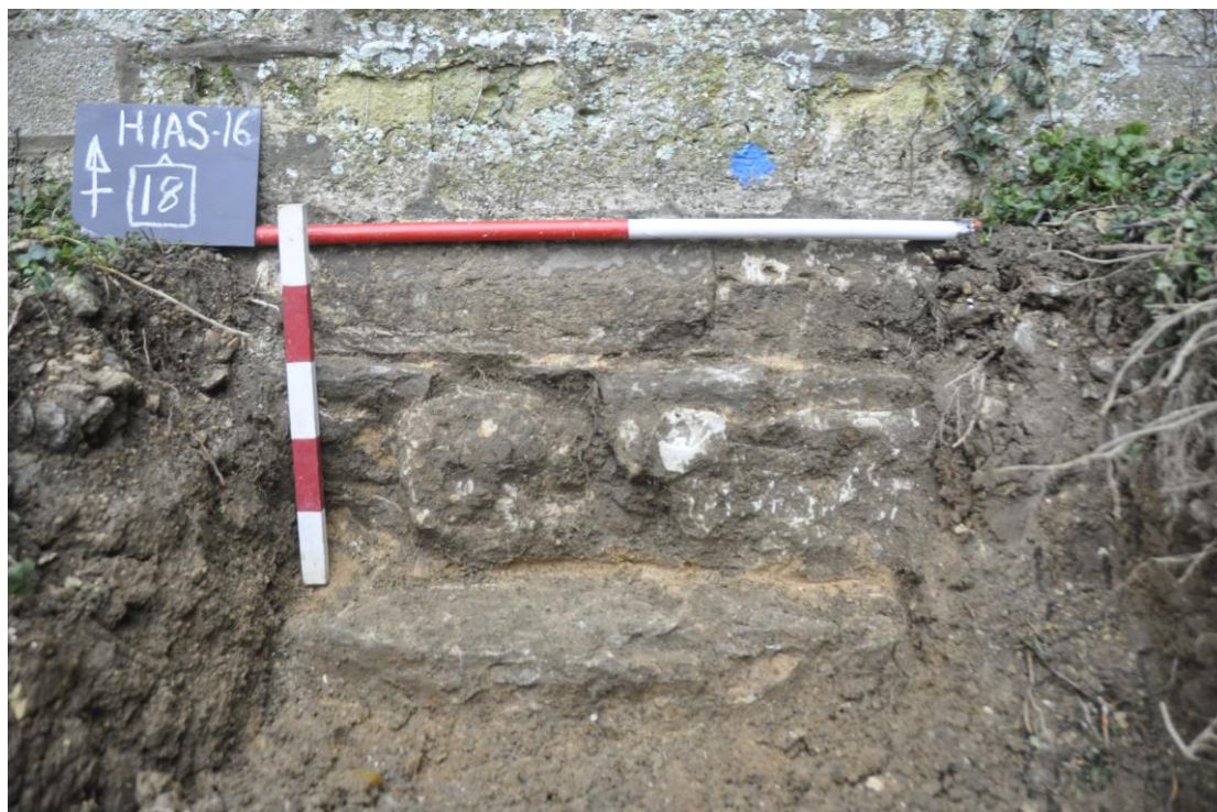
Plate 5. Southern, external foundations (18) of tower. Note stepped foundation and chamfer course. View to north.
